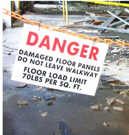
Figure 2-2. Warning sign on the operating floor.
