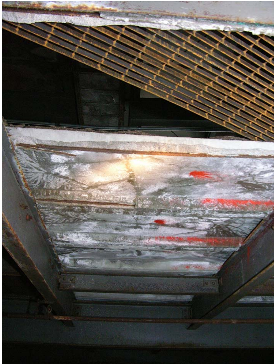
Figure 3-2. Degraded floor panels and the accident scene viewed from the pipe gallery catwalk below.
