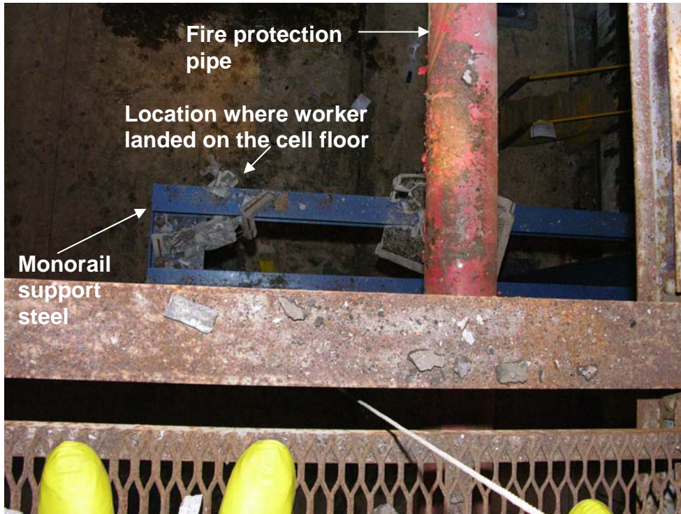
Figure 2-5. Accident scene – view looking down from the pipe gallery catwalk.
