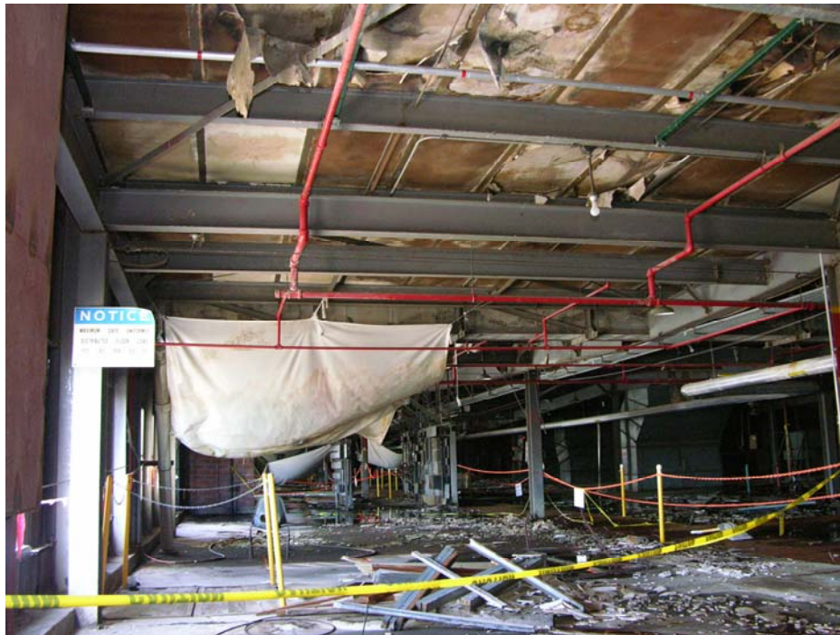
Figure 3-6. Deteriorated roof viewed from the operating floor.
