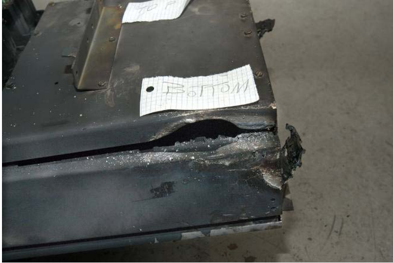
Figure 2-6. Back of switch 3A bus cover plate
