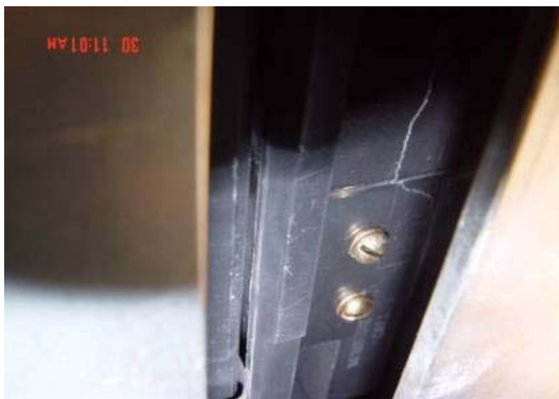
Figure 2-13. Crack developing in ABS base of switch not involved in the accident
