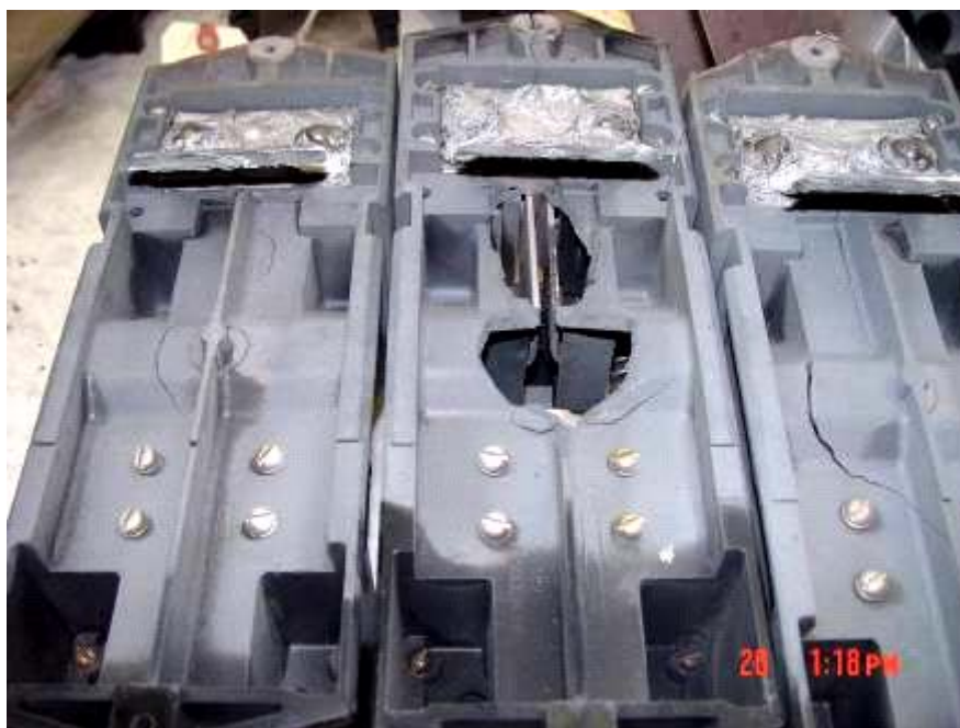
Figure 2-11. Switch 3A ABS base Phase B displaced piece
