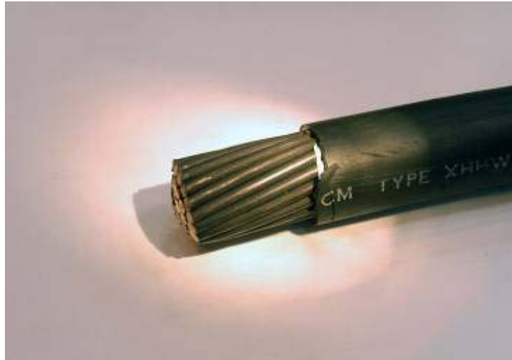
Figure 2-14. Damaged cable which was underwater in manhole from substation 6C to panel PB-1
