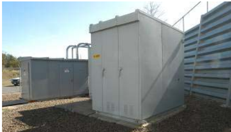
Figure 2-3. Substation 6C outside Building 1006A
