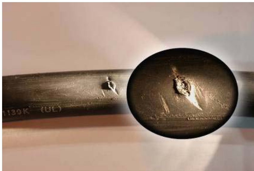
Figure 2-15. Damaged cable with oxidized copper
