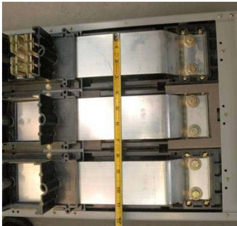
Figure 2-7. Undamaged bus on undamaged switch
