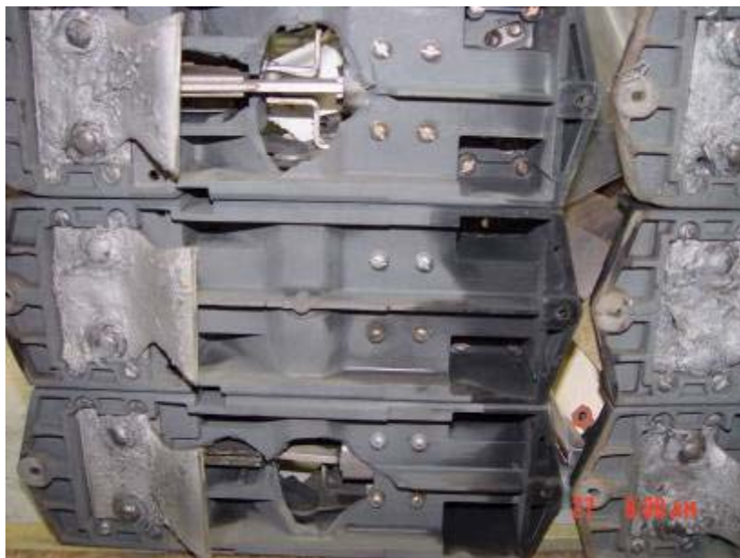
Figure 2-12. Switch 2A ABS base Phase A and C displaced pieces (Only one contact clip could be found)
