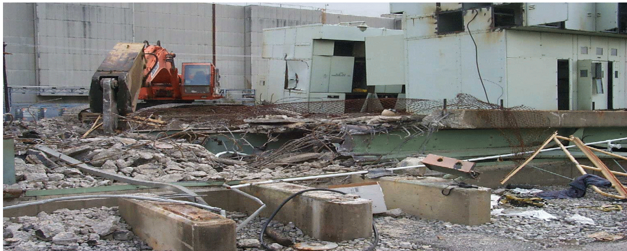
Exhibit 2-2. Near View of Accident Site at Building K-791 North Job Site (from W to E).
