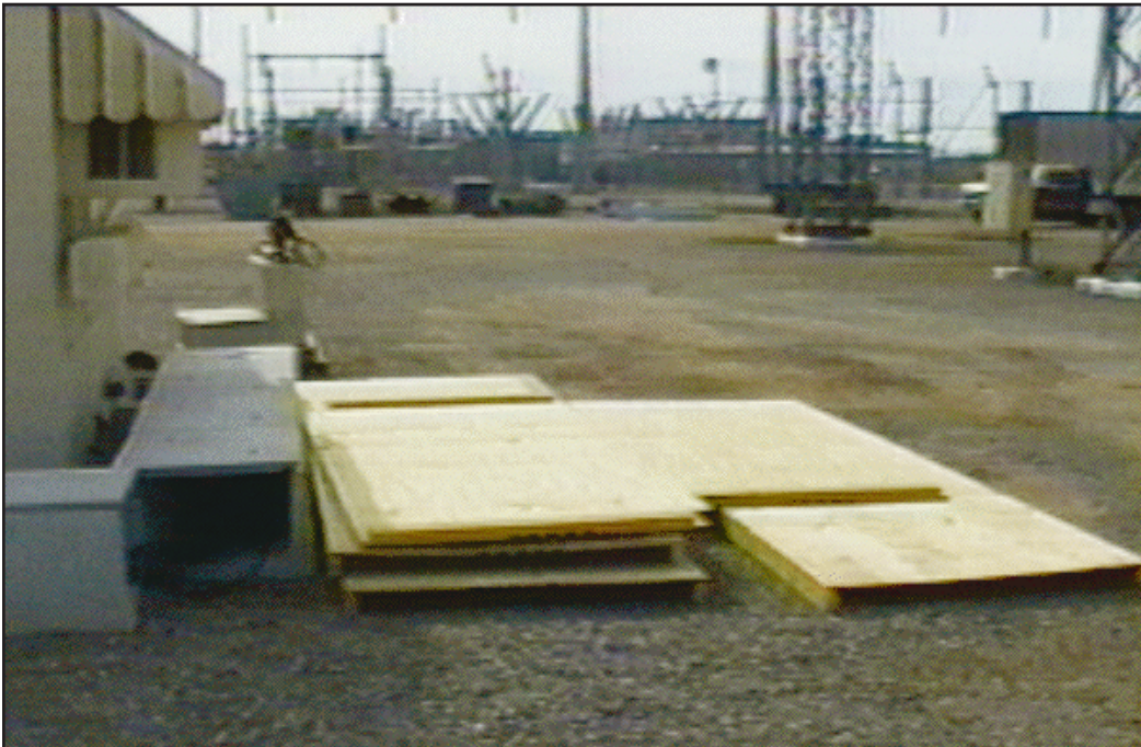
View of the prefabricated isolating barriers to be placed along the south and west sides of the 12.47-kV bus structure
