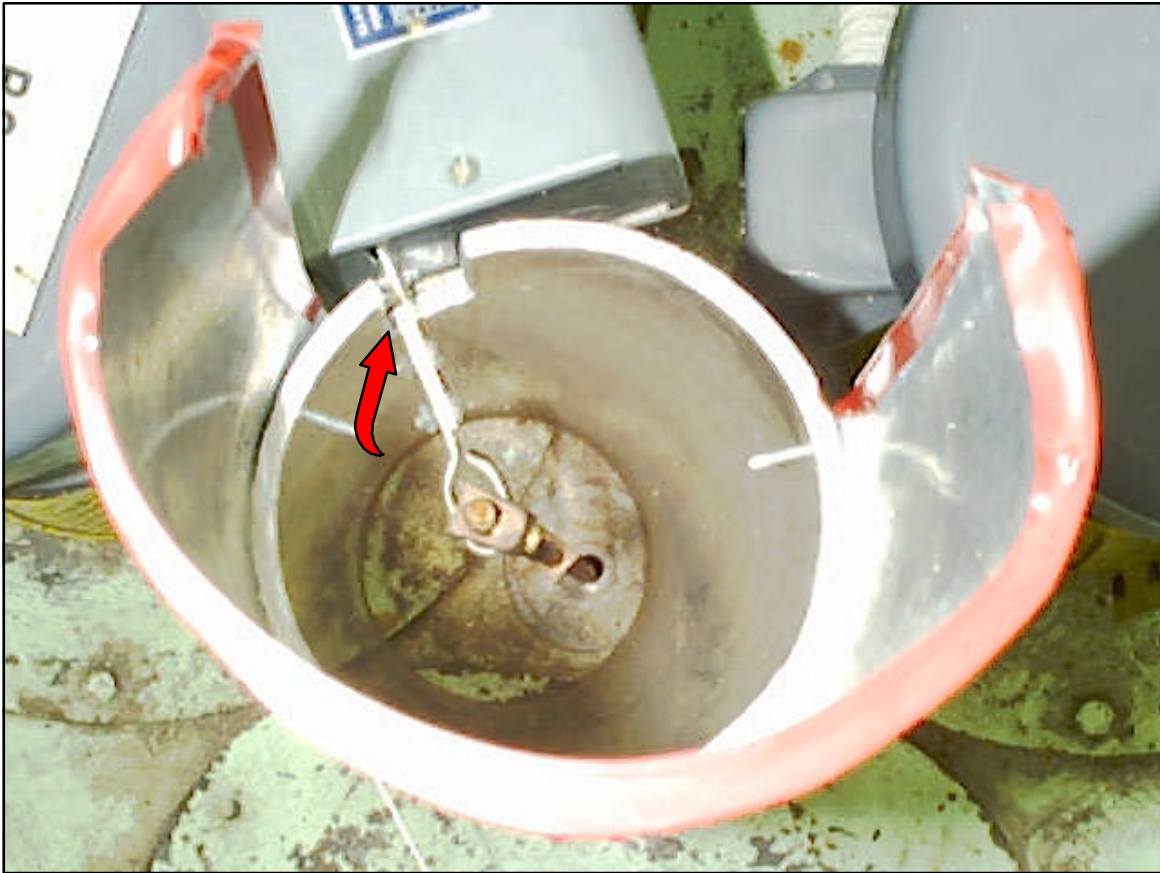
Figure 12: Actuator arm for sump pumps
