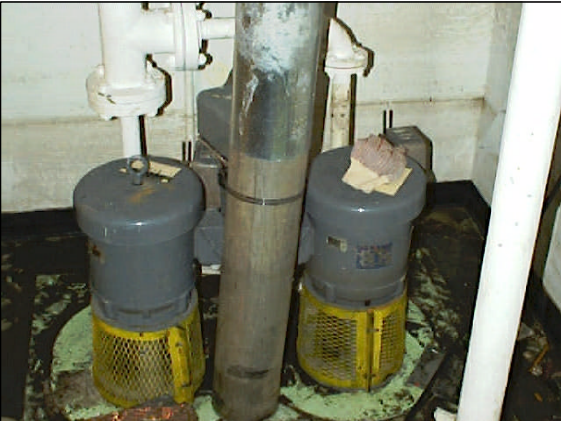
Figure 3: Sump Pumps (PS-1 & PS-2)
