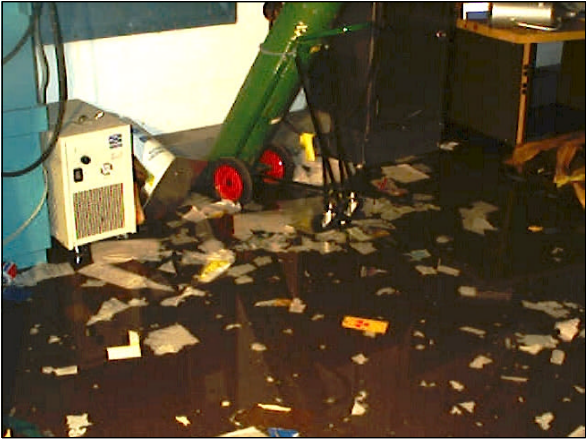
Figure 9: Debris floating in sub-basement with one inch of water
