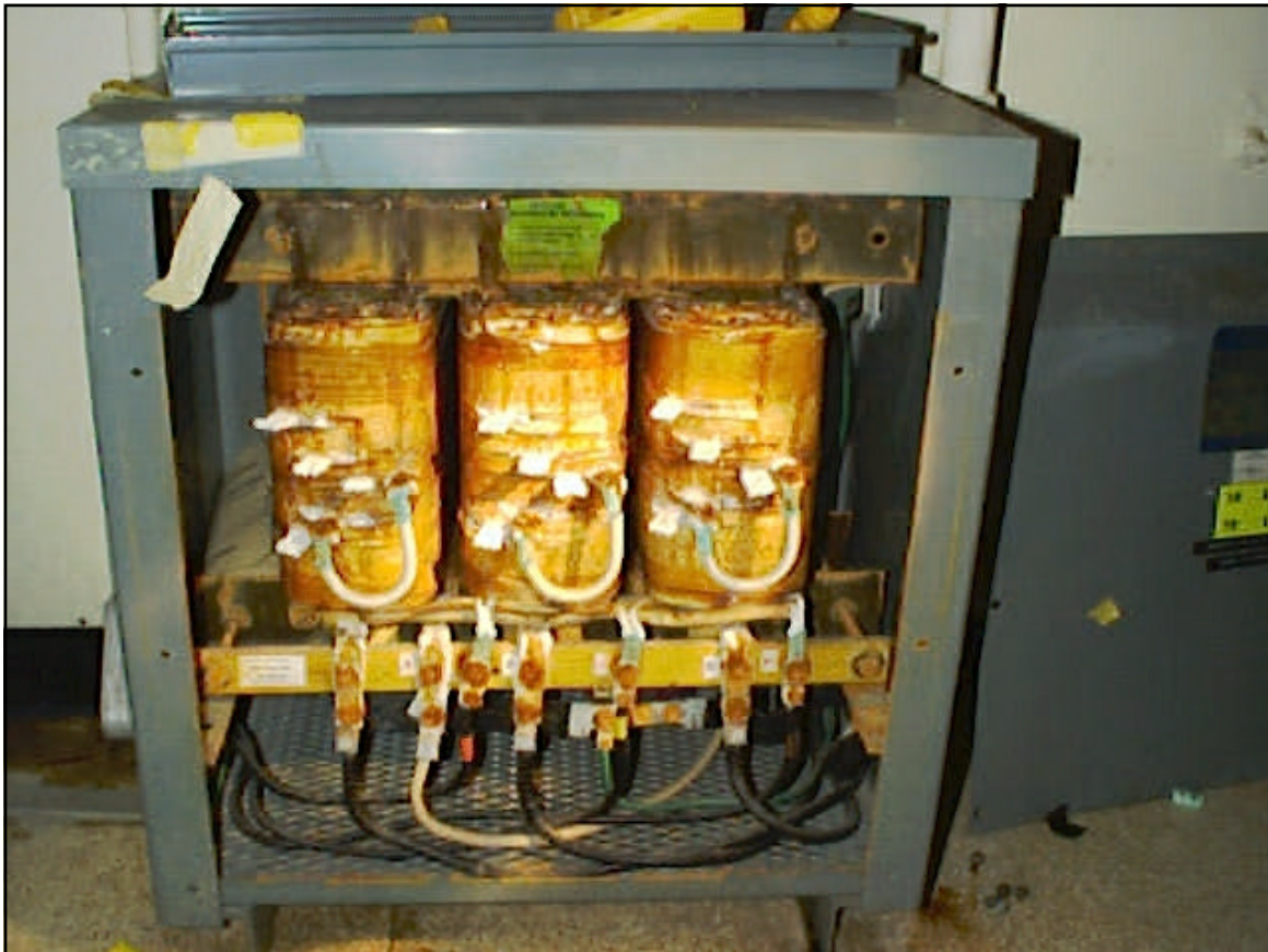
Figure 10: Damaged transformer in sub-basement
