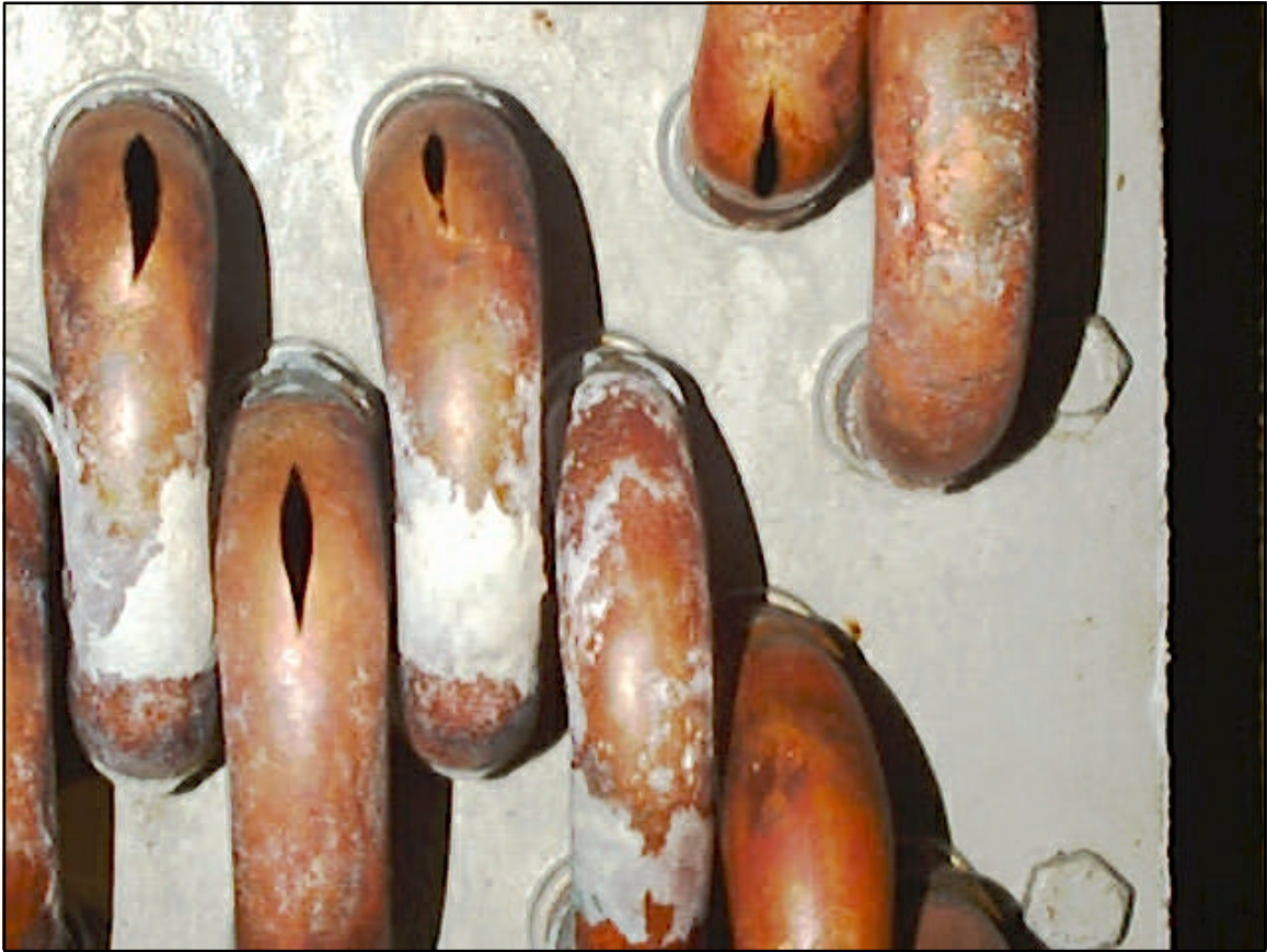
Figure 4: Ruptured Coils of CWE-1
