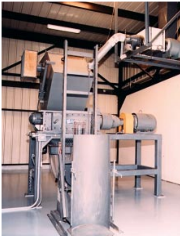
Exhibit 2-1: Shredding Unit in B-513 (prior to dry run).
