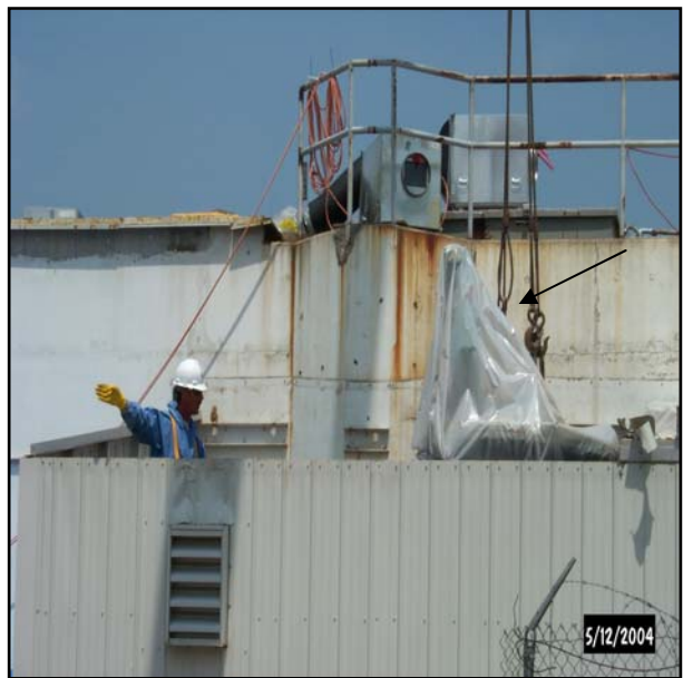
Figure 2-3. Mixer for Tank T-12 Extends Beyond the Roof of the T-13 Annex
