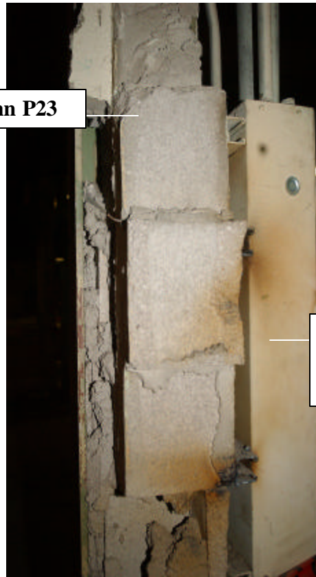
Exhibit 2-5. View of Column P23 with Block Remaining in Column after Wall Demolition (Looking South)
