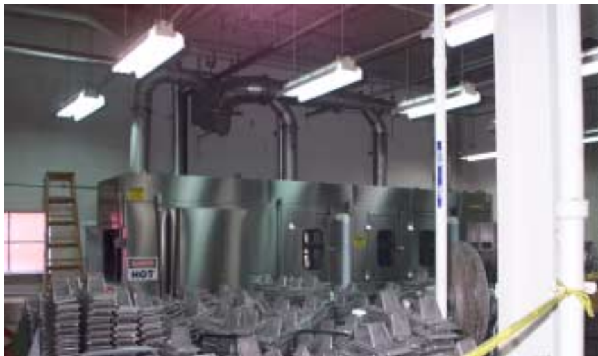
Exhibit 3-1. Exhaust Fan and Motor above the Tunnel Washer
