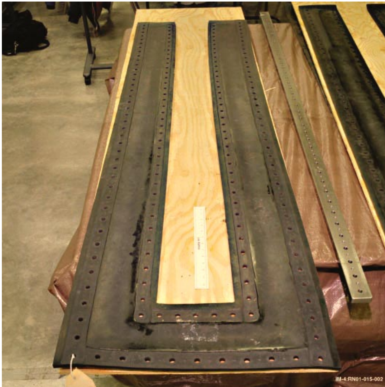
Figure 9. The right Rear Tri-Plate Gasket and one of the backing bars after removal. The gasket displayed significant deterioration along borders where the backing bars were attached
