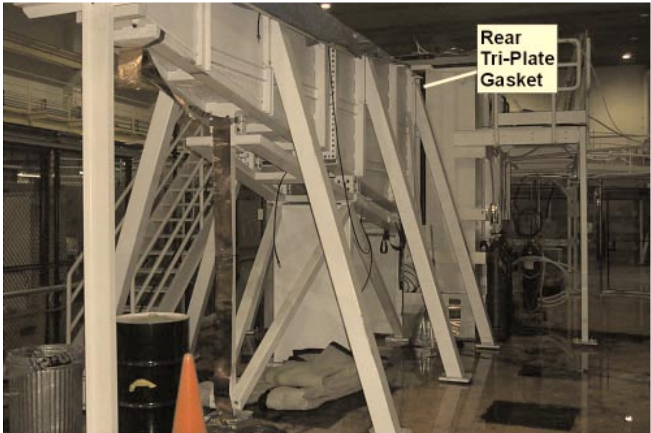
Figure 3. The First Article Assembly, where the leak occurred, is composed of the Maintenance Unit Tank and the Vertical Transmission Line Tank (note oil on floor).
