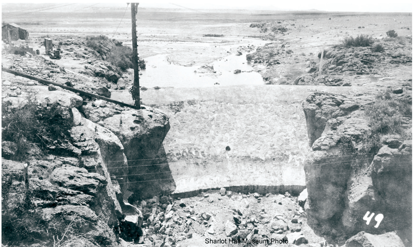
Figure A7. Photographs showing construction of Sullivan Lake Dam, circa 1936. View is west. Sluice box in upper photo was used to divert perennial flow around the dam. Exposed rocks in gorge near the dam are 4.5 Ma basalt flows. Sullivan Buttes shown at skyline in upper photo. Note sediment filling channel upstream of the dam.
