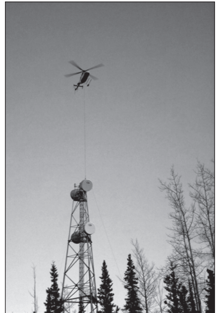
The Bell-407 pilot demonstrates extreme proficiency while placing an antenna on a tower. Photo by Tim Graves, Air Logistics, Inc.
