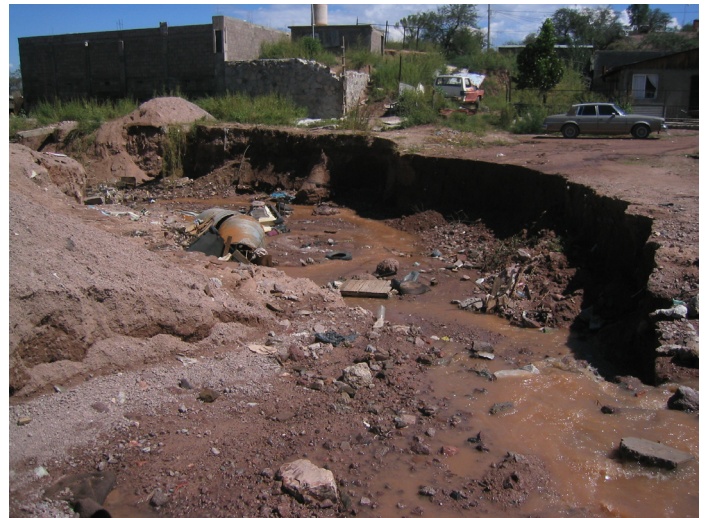
Figure 5. Overflow from La Represa erodes soft sediments which impact El Tecnológico wash.
