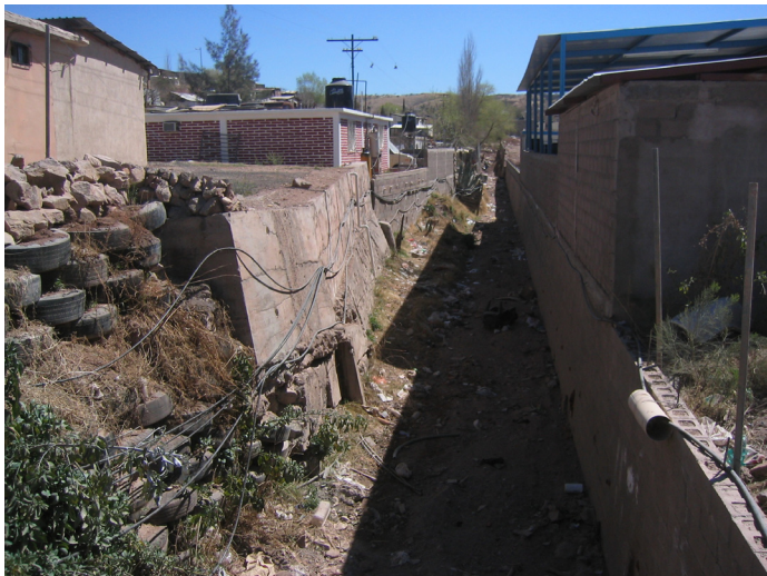
Figure 4. Floodplain encroachment and channelization (Colonia Virreyes).
