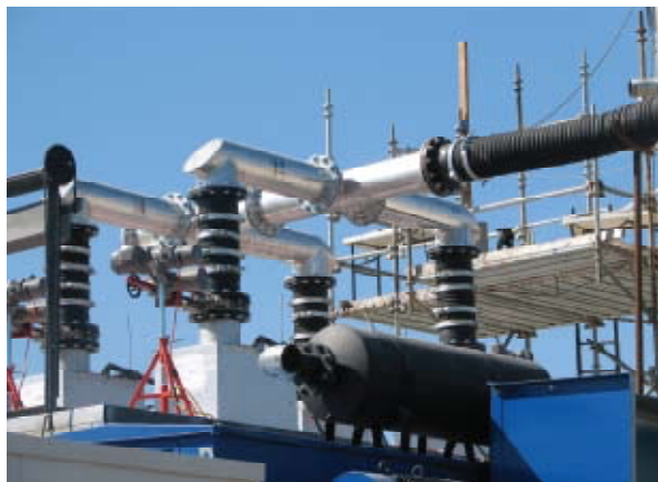
Figure 2-5. Feed Distribution System
