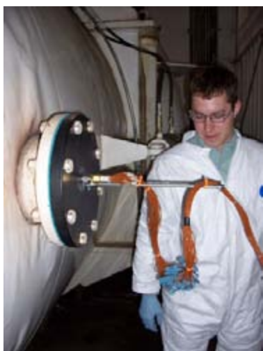
Photo 23. Connectors Not Inverted Allowing Condensate to Collect in the Connectors
