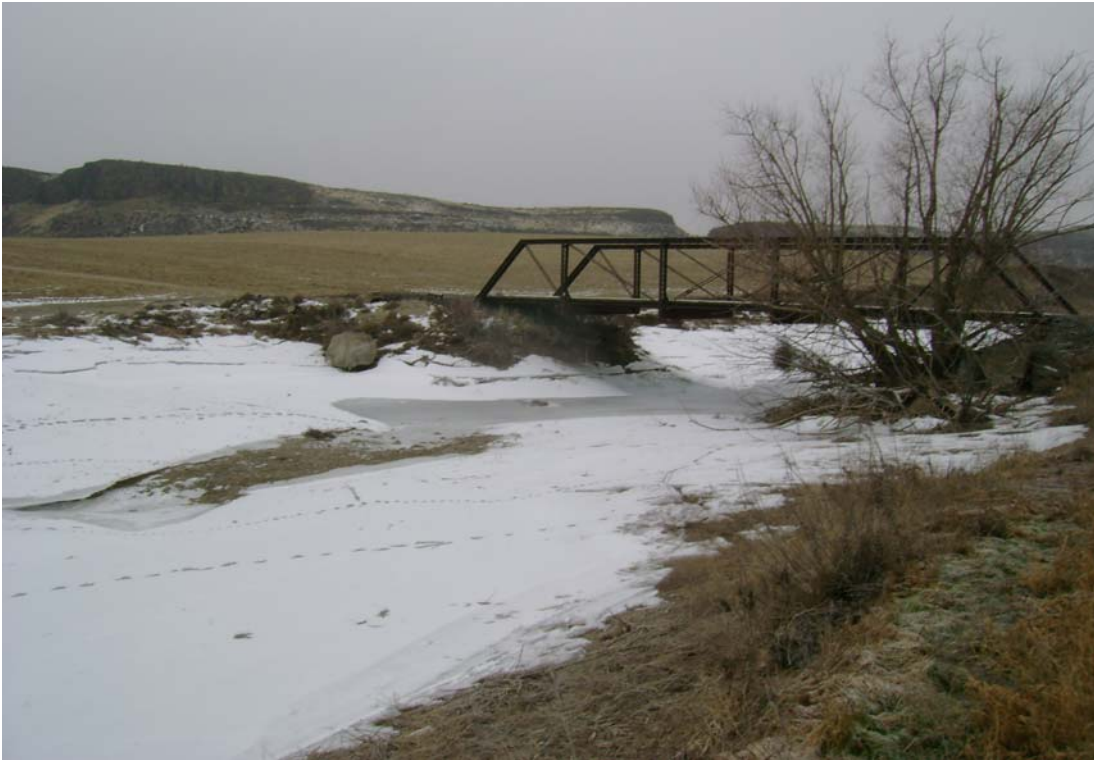
FIGURE E-6 Sample photo documentation of bridge features and high water marks
