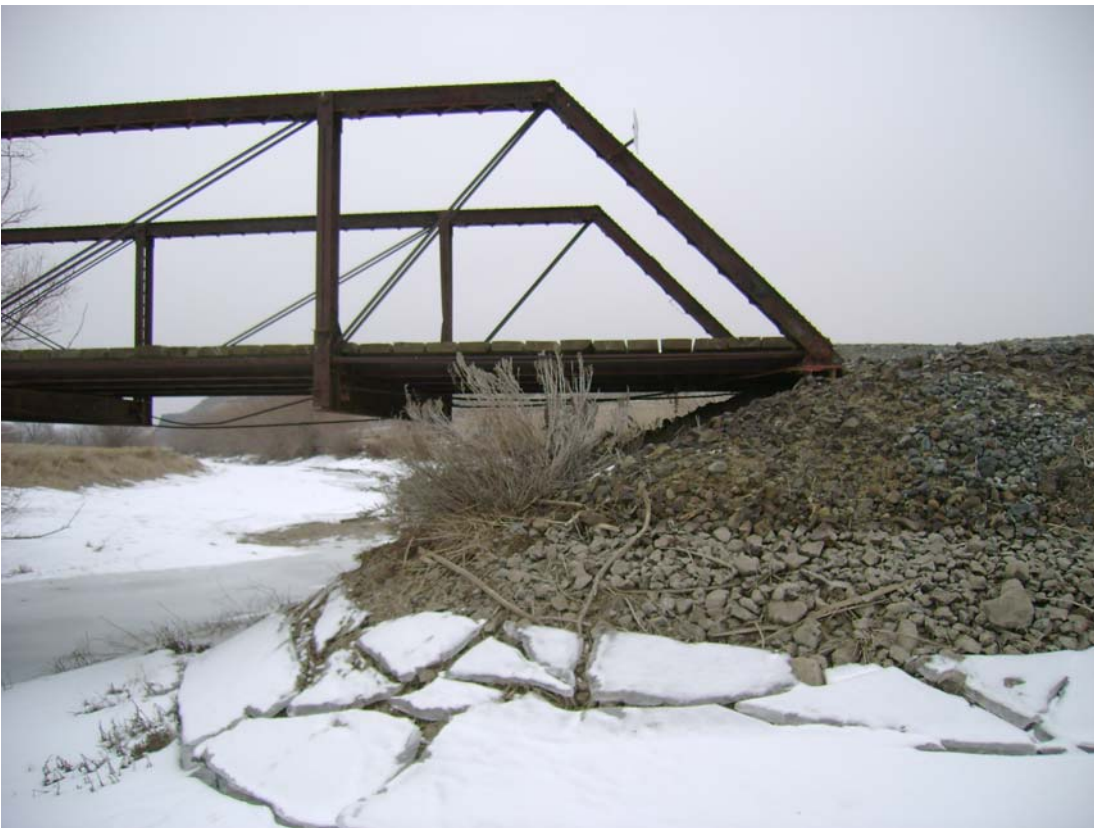
FIGURE E-7 High water mark at the "Private Bridge"
