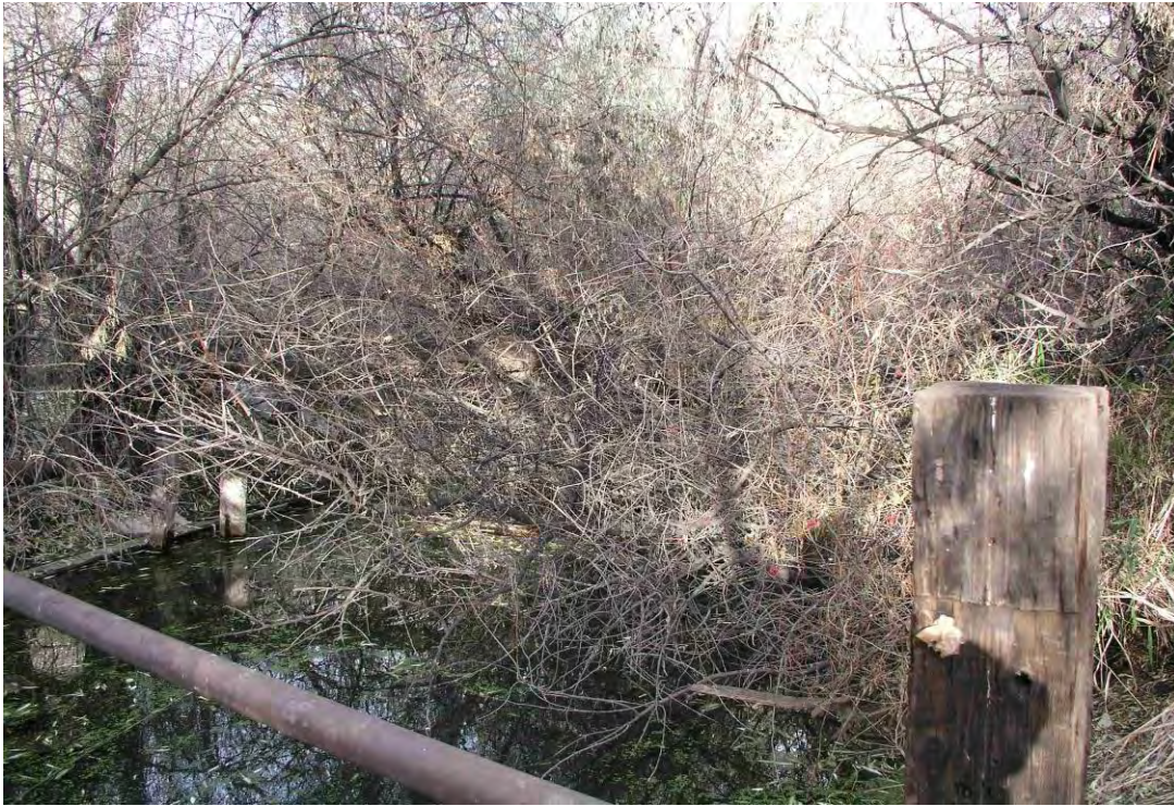
Figure 10. Drains on the Oxbow property are lined with dense stands of trees and brush.
