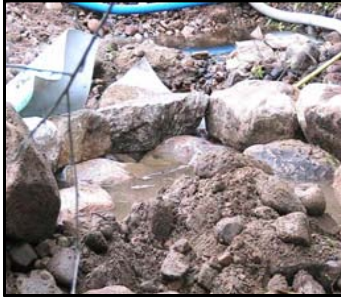
Photo A-9. Looking upstream at base rocks of Weir No. 1. To prevent downstream movement, the rocks on the top layers are behind the base rocks.
