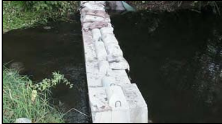
Photo A-17. Concrete “ecology blocks” were used as the core of Cofferdam B, which dewatered the construction sites for Weirs No. 2 and 3. They are cast from leftover concrete batches, reducing waste; note the rebar “lifting eyes” for placement and removal.
