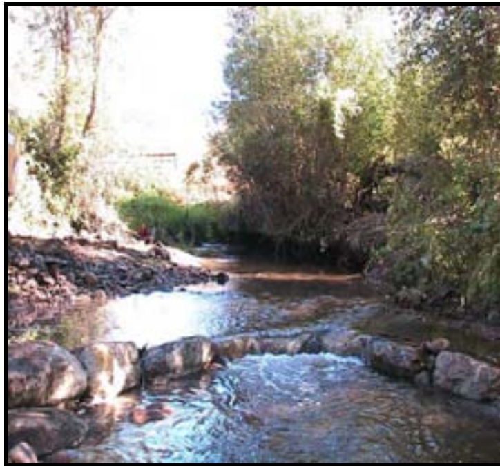
Photo A-16. Looking upstream at Weir No. 1 after Cofferdam A has been removed.
