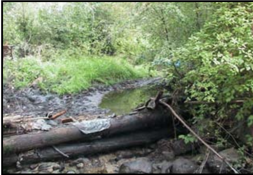
Photo No. 19. The Lower Stokes Diversion Dam was deconstructed in stages to facilitate electro-shocking and removal of fish from project area.
