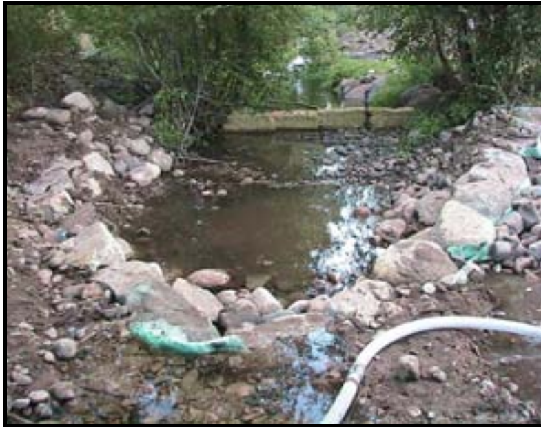
Photo A-11. Looking downstream at completed Weir No. 1 (trash pump hose in foreground).
