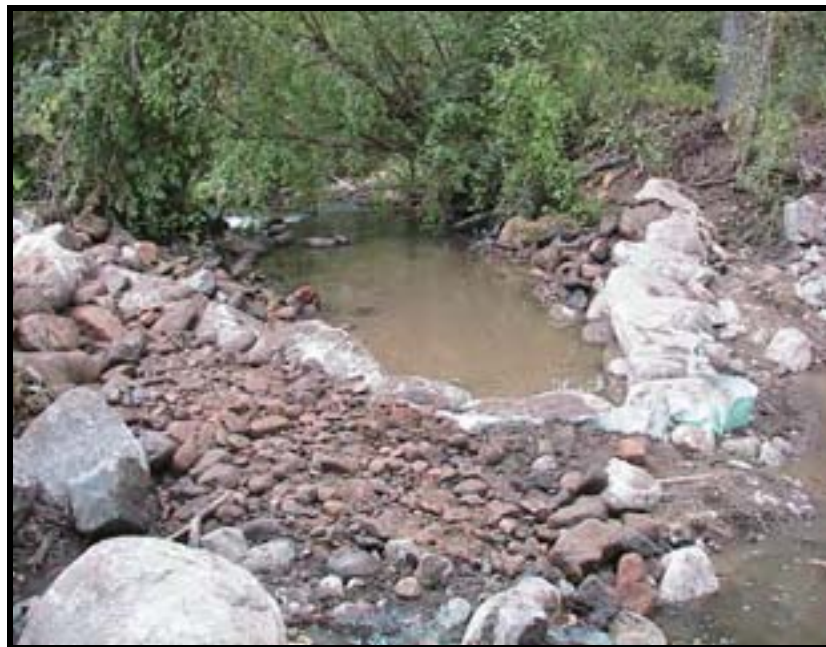
Photo A-22. Looking downstream at Weir No. 3 about 3 hours after Photo A-21 above was taken. The weir has been backfilled and the scour hole excavated.
