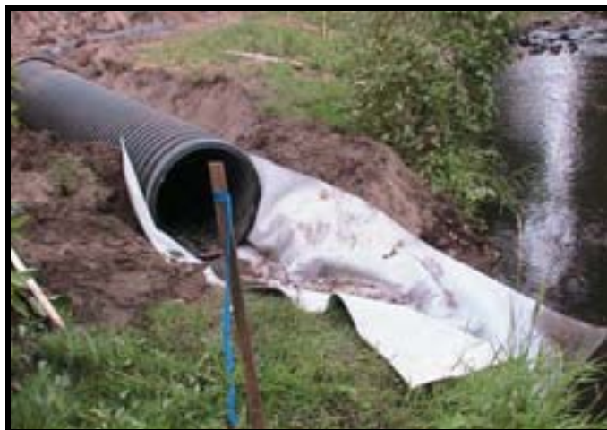
Photo A-6. Downstream end of dewatering pipe with fabric for erosion control.
