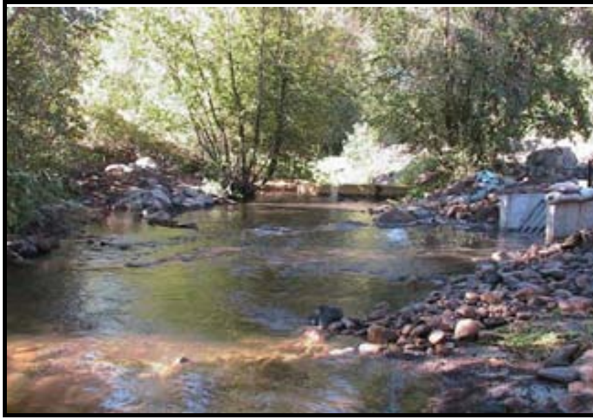
Photo A-15. Looking downstream at Weir No. 1 (center) from the remains of Cofferdam A. The new diversion box is at center right.
