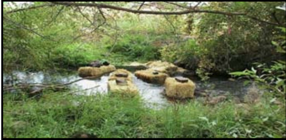
Photo A-7. Straw bales below Weir No. 1 construction area prior to dewatering. The straw bales help filter silt during and after construction.
