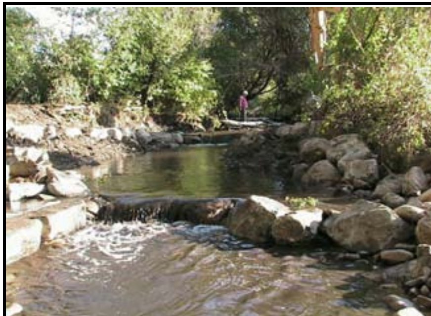
Photo A-24. Looking upstream at Weirs No. 3 and No. 2 as water muddy from the removal of Cofferdam B flows past.
