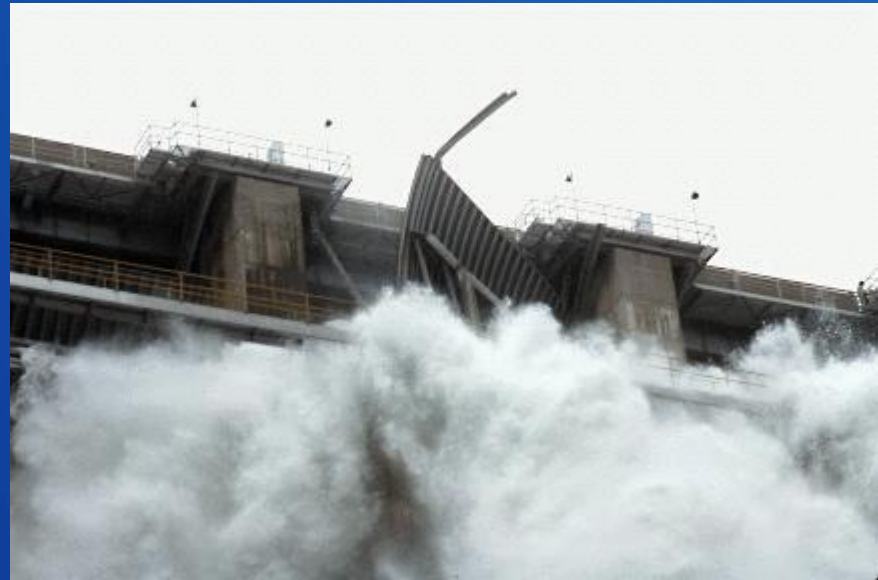
Photo: 1995 Folsom Dam Spillway Gate Failure
