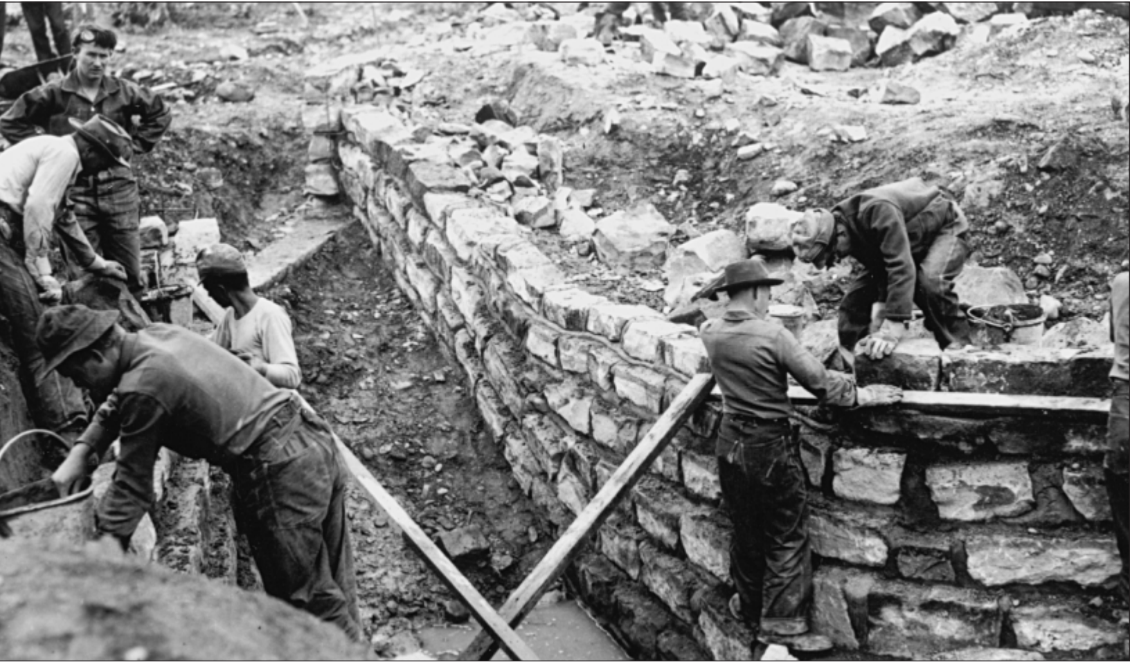
An irrigation canal wall being hand constructed by men of the Montrose CCC camp, April 21, 1941. The CCC program of the Great Depression taught skills to men who otherwise would have had difficulty learning trades and supporting themselves in the jobless market.
