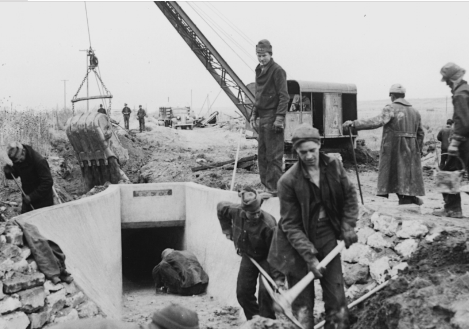
A mechanical dragline works alongside men with hand tools in construction of a "pipe siphon" near Montrose, Colorado, February 9, 1940. Within two years, the Civilian Conservation Corps would be shut down, with most of its resources—human and otherwise—transferred to the war effort. Men of the Montrose CCC unit were taught the fundamentals of excavation, form-building, concrete reinforcement, road construction, and quarrying—abilities which many of them later carried into civilian life.
