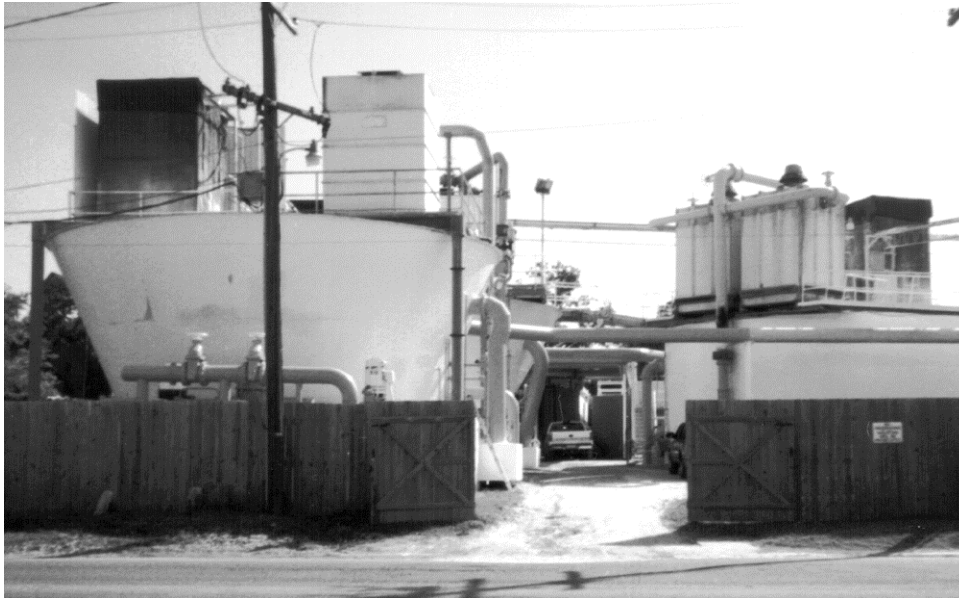
Figure 2-3 – Forced-Draft Tray Aerators
