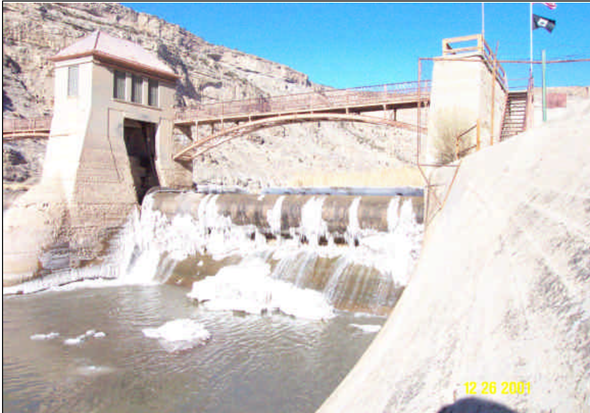
Figure 3 - Left bank (Interstate 70 side) roller gate at the Grand Valley Project Diversion Dam (Photo Dated Winter 2000)
