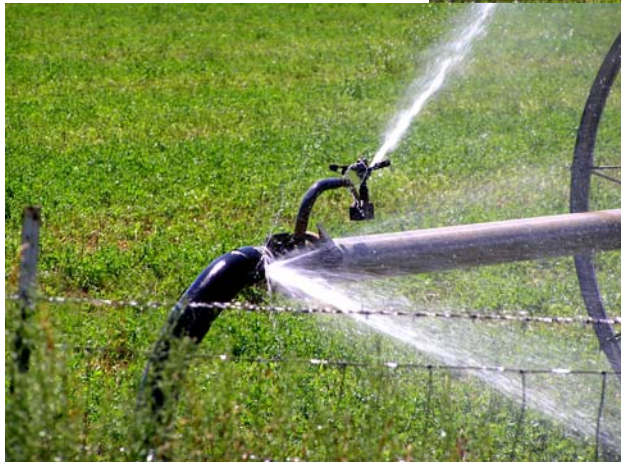
Figure 26, Hose leaks are rare but prolific and expensive to repair
