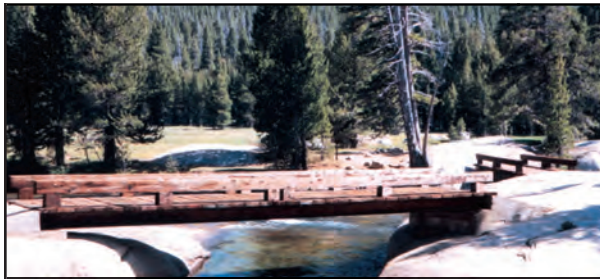
Figure 16 (above): Site 8: Bridge, Lyell Fork of Tuolumne River. This will be a standard bridge installation.
