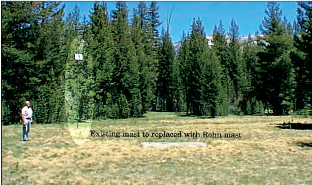
Existing antenna mast will be removed and the new mast will be placed in the same location. A hole 1.5 feet diameter by 3 feet deep would be dug for the base of the Rohn mast.
