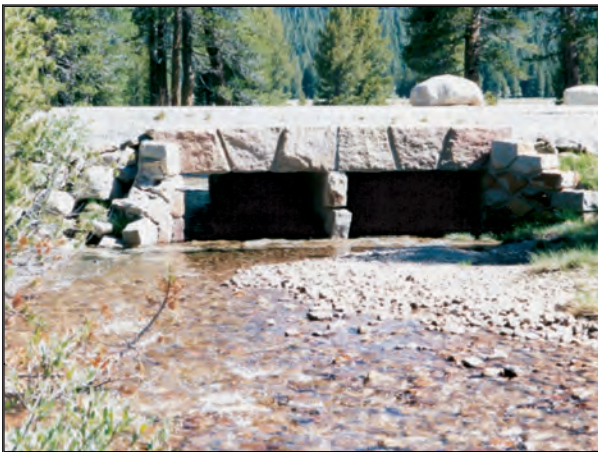
Figure 11: Site 4: Tioga Road culvert at Unicorn Creek. This will be a standard culvert installation.
