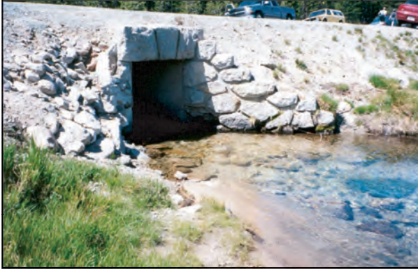
Figure 10: Site 3: Tioga Road culvert at Budd Creek. This will be a standard culvert installation.
