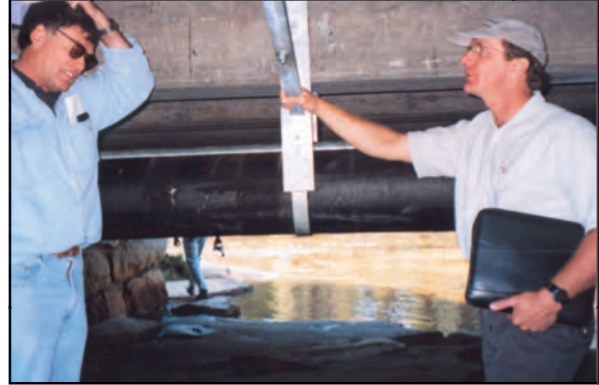
Figure 12: Site 5: Tioga Road Bridge, Tuolumne River. Dan Cayan and Mark Butler examine the underside of the bridge, where data-logger will be housed
