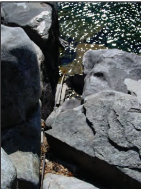
Photo 3: Old gage site. The instrument package will be deployed next to an existing pipe which will provide an anchor structure for communications cabling.
