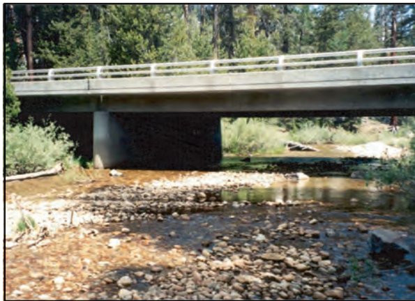
Figure 8: Site 2: Tioga Road bridge across Yosemite Creek. This will be a standard bridge installation.
