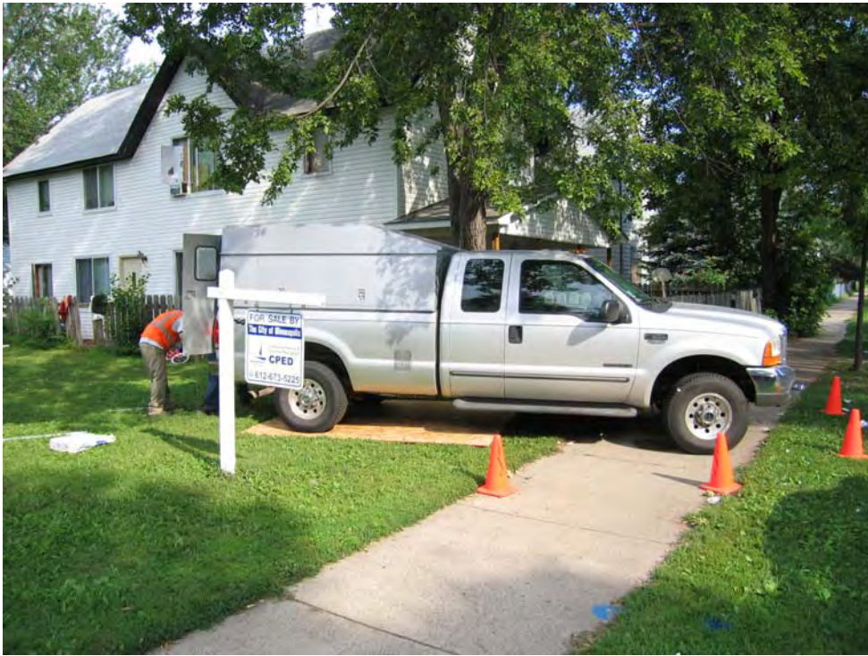
Figure 1: View of typical Geoprobe rig setup. Note: construction cones and usage of plywood to prevent compaction and rutting of lawn.
