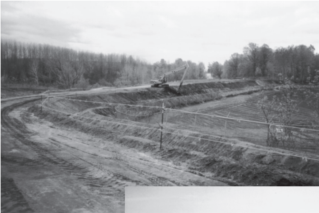
(To the left) A berm and ditch has been constructed around Tar Lake to control runoff.
