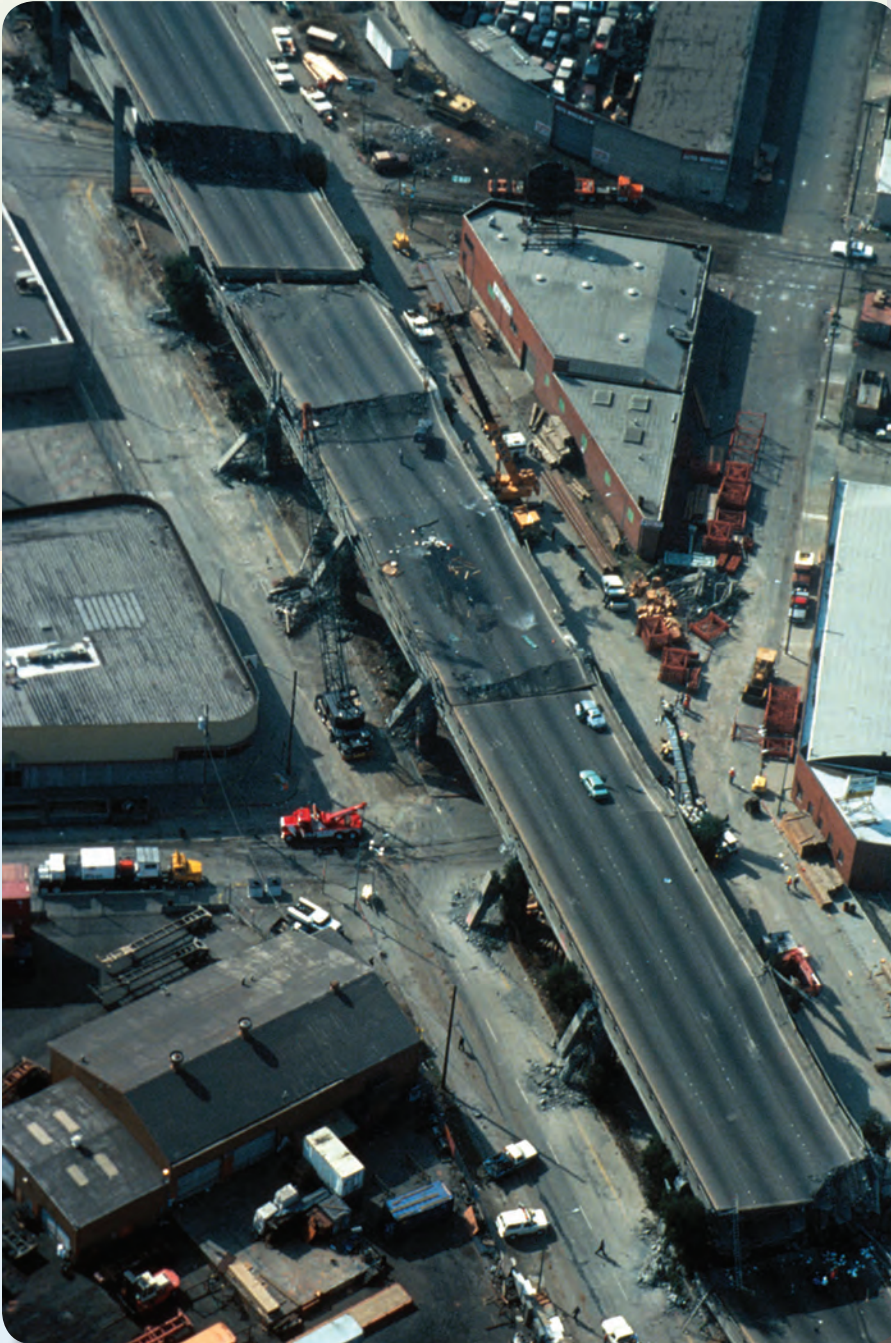
Collapsed section of the Cypress viaduct of Interstate 880 in Oakland following the magnitude 6.9 earthquake in 1989 in Loma Prieta, California.
