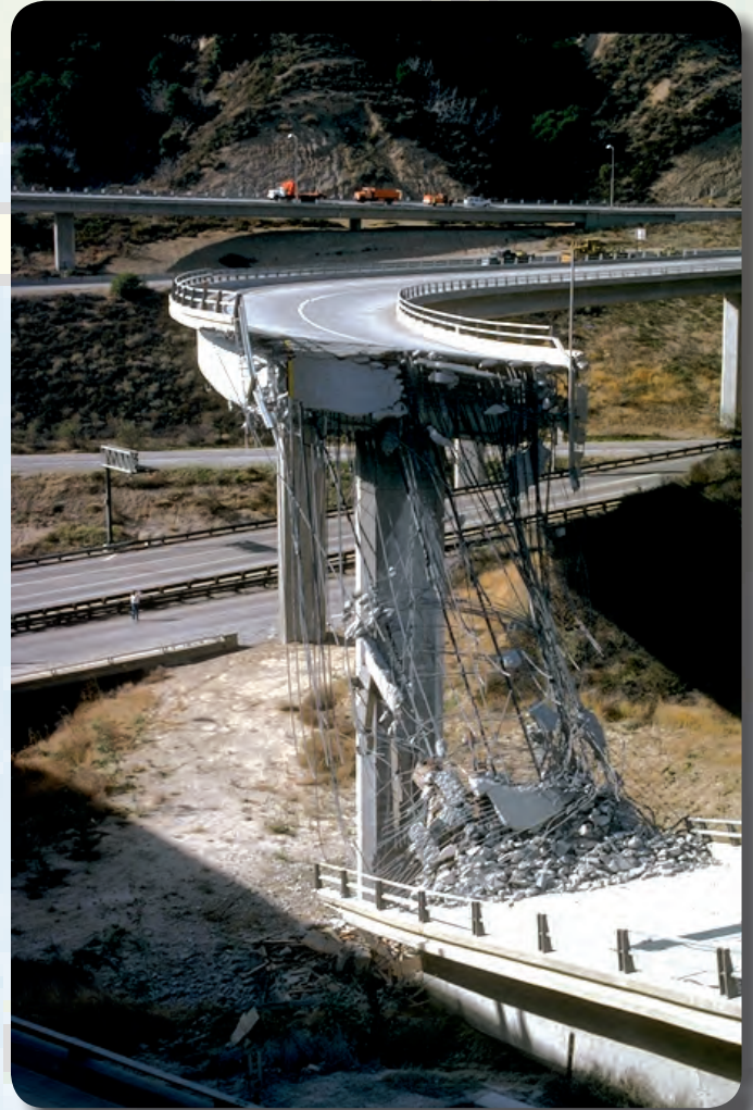
Collapse of the Interstate-5/State Highway-14 interchange showing damage north of Los Angeles caused by the 1994 magnitude 6.7 Northridge, California, earthquake. Thousands of State and County bridges were shaken at varying intensity levels during this earthquake; many required inspections.
