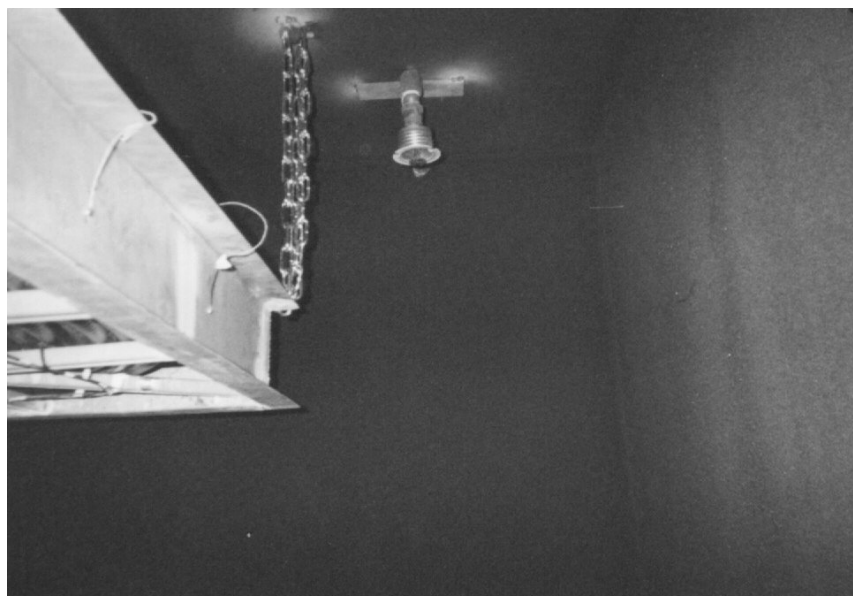
Figure 4-7. Water sprinkler head inside fire test cell.
