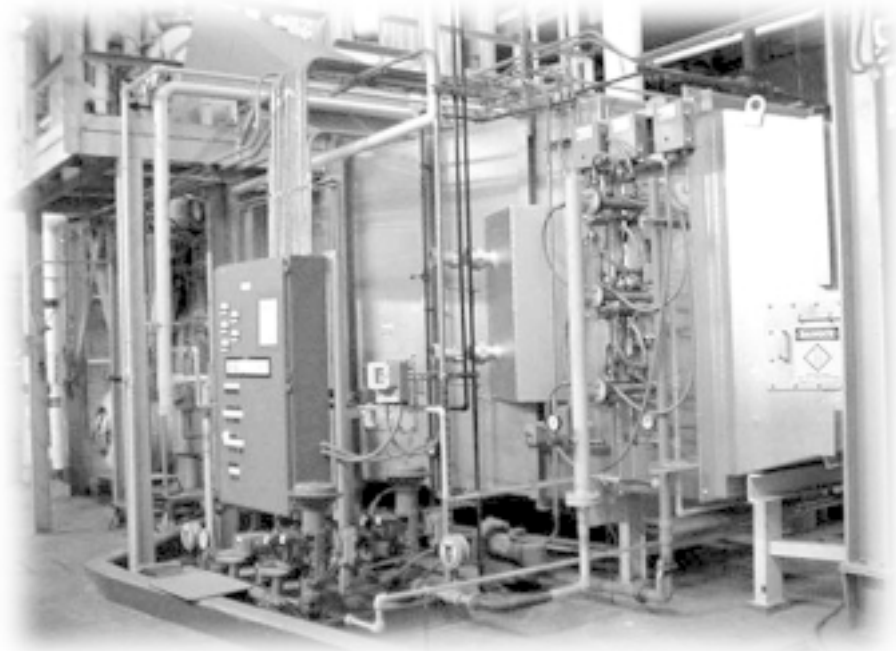
Heat recovered from the combustion turbine is utilized in a 50,000 pound per hour boiler.
