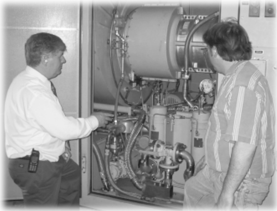
The 5-MW Taurus 60 from Solar Turbines, Inc. logged 18,000 hours of operation over its first 3 years. Installation went smoothly, thanks to the contractor.
