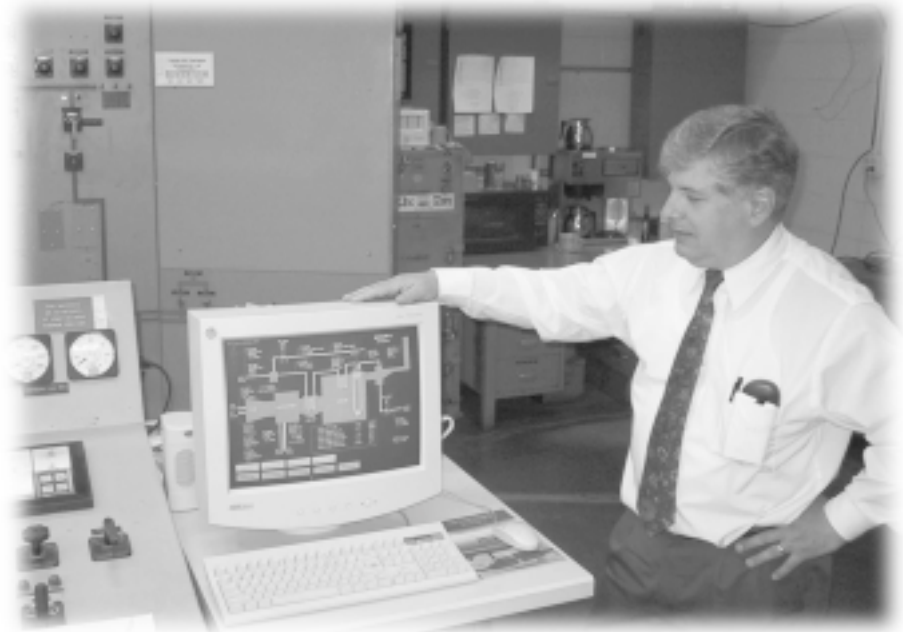
The control room monitors the operating conditions of the combustion turbine and heat recovery system.
