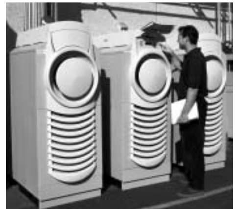
Capstone Turbine Corporation/PIX08130
