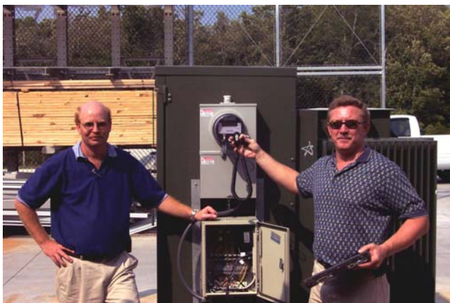
Figure 8. Lewis Shaw and James Green (BEMC) Connecting Simulator to Lowe's Meter
