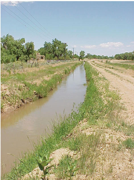
An unlined canal near Paseo del Norte in northern Albuquerque. Such canals are now represented in the ground-water-flow model with variable leakage rates.
