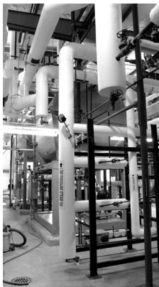
A view of the steam condensate and boiler water treatment equipment in Building 359.
