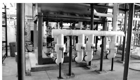
The pumps used in the condensate and boiler water treatment equipment in Building 359.
