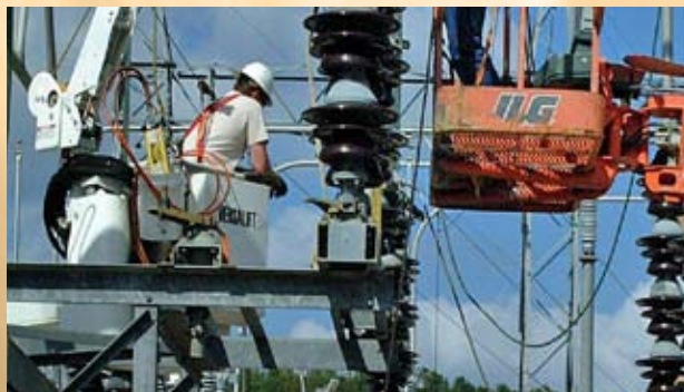
Substation Work, Southwestern Power Administration.
