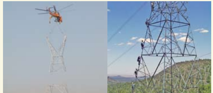
Transmission Towers at Western Area Power Administration.
