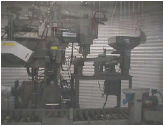
Figure 2-3: Drum Venting Equipment
