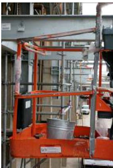
Figure 1. Manlift proximity to upper I-beam
