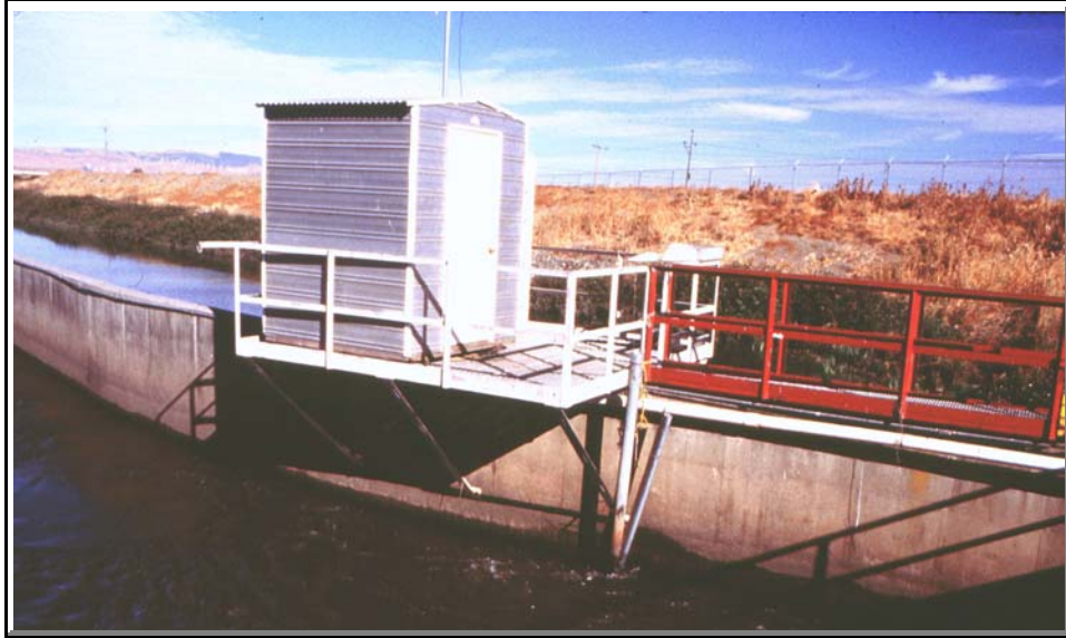
Figure 3a.—Calibration shed behind the intake screen at the TFCF. The Datasonde was installed in the pipe located adjacent to the shed platform.
