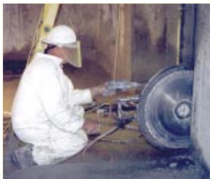
Energy Technology Engineering Center technician uses a diamond concrete cutting saw to cut thin slices along the affected concrete seams to avoid creating additional waste.
