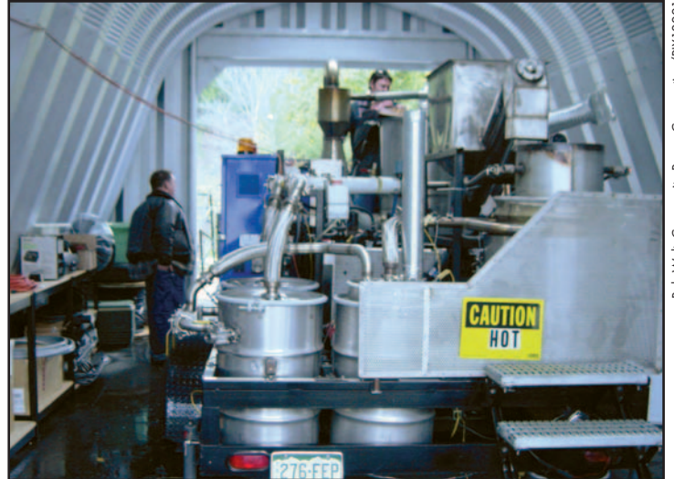
Small modular unit connected to a power line.
