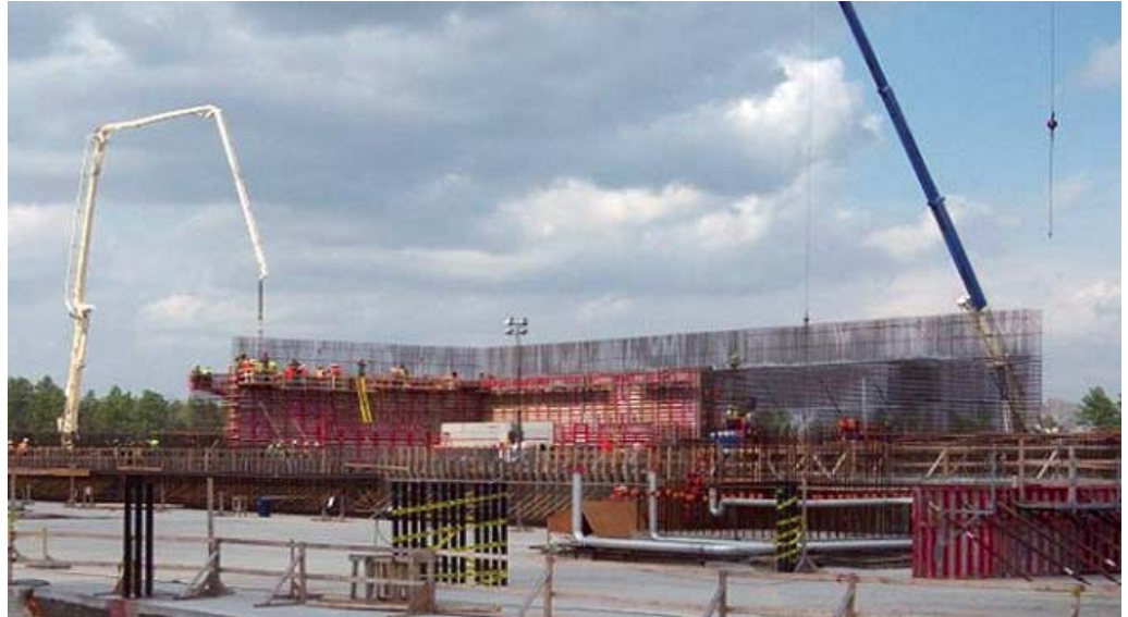
CONSTRUCTION ON SCHEDULE: Exterior walls of the Fuel Manufacturing Building being erected (April 2008).
