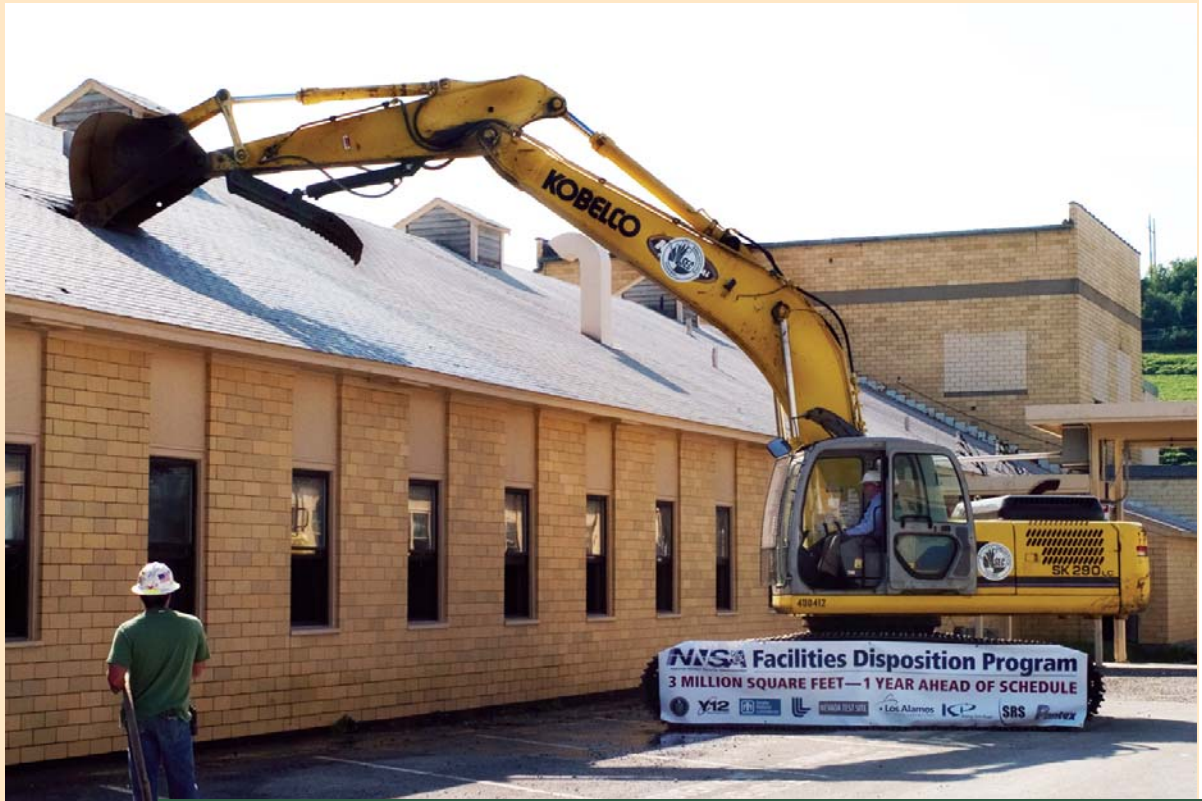
TERMINATOR: Deputy Administrator William Ostendorff operates a hydraulic excavator to begin razing an old building at the Y-12 National Security Complex.
