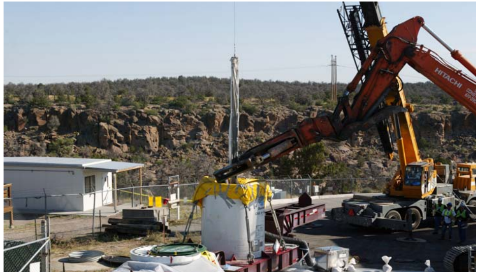
LANL TA-54 CLEANUP: Seven "stringers" formerly used to push targets in and out of a linear accelerator beam line for radioisotope research at Los Alamos National Laboratory have been safely removed from the lab's Technical Area 54. The twenty-six foot long hollow steel rods filled on the lower end with cement, sand, and lead were transported to a permitted treatment and disposal site in Utah. Removal of the stringers is part of the proposed closure plan for the Material Disposal Area L.
