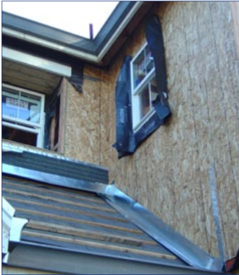
Installing window and roof flashing is critical for long-term durability and must happen at the correct stages of construction.
