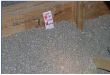
Researchers from Washington State University are evaluating how the bumps and vibrations of highway travel affects the settling of attic insulation installed in the factory.
