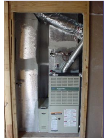
A fresh air intake duct with a Constant Airflow Regulator runs from the outside to the return plenum. The furnace operates continuously on low speed to provide whole-house ventilation.
