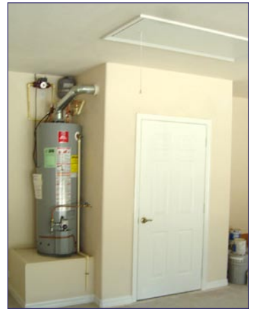
FIGURE 17: Air Handler in Conditioned Space
