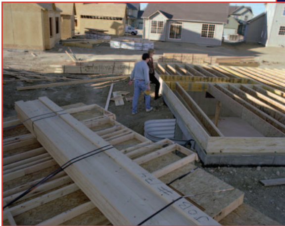
Prefabricated wall panels await assembly at the Meadow View community in Longmont, Colorado. McStain Enterprises is the builder partner (IBACOS).
