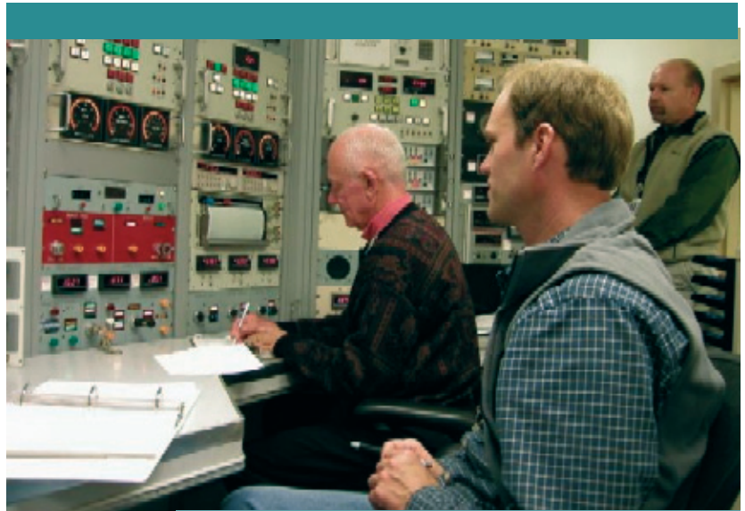
REACTOR CONTROL ROOM: Sandia SPR reactor operators monitor the operation of the SPR III reactor in the control room while an NNSA Sandia Site Office facility representative looks on.
