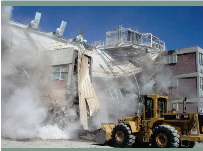
COMING DOWN: Demolition efforts are underway for a 1960s-era building at Sandia National Laboratories in New Mexico.
