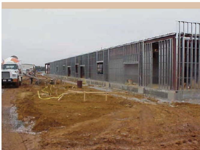
GOING UP: A new administrative and classroom building for the Office of Secure Transportation’s Eastern Command is under construction in Tennessee.
