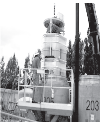
Lawrence Livermore National Laboratory Decontamination and Waste Treatment Facility are loading drums with radioactive waste into a TRUPACT II container for shipment offsite.
