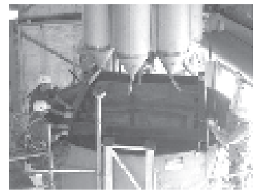
Pulse Jet Mixers at the Waste Treatment Plant located at the Hanford Site.
