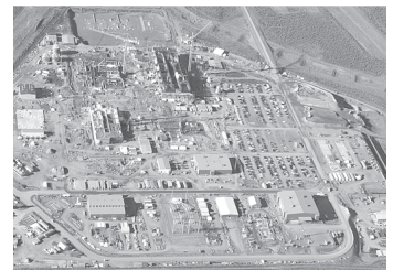
An aerial view of the Waste Treatment and Immobilization Plant construction site.
