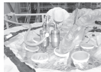
Workers at the Sludge Retrieval and Disposition Project connect hoses to ports in the top of large diameter containers that will hold sludge from the North Loadout Pit in the K East Basin at the Hanford Site.
