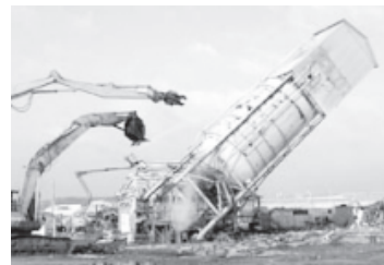
A view of the Bulk Lime Handling building as it toppled to the ground.
