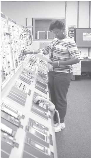
H Area Canyon Control Room at the Savannah River Site.
