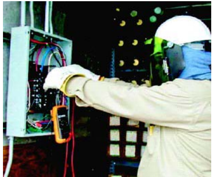
An electrical worker checks an energized panel while wearing appropriately rated flash PPE for 240v or less
