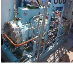
CNG Compressor Lube Reciprocating
