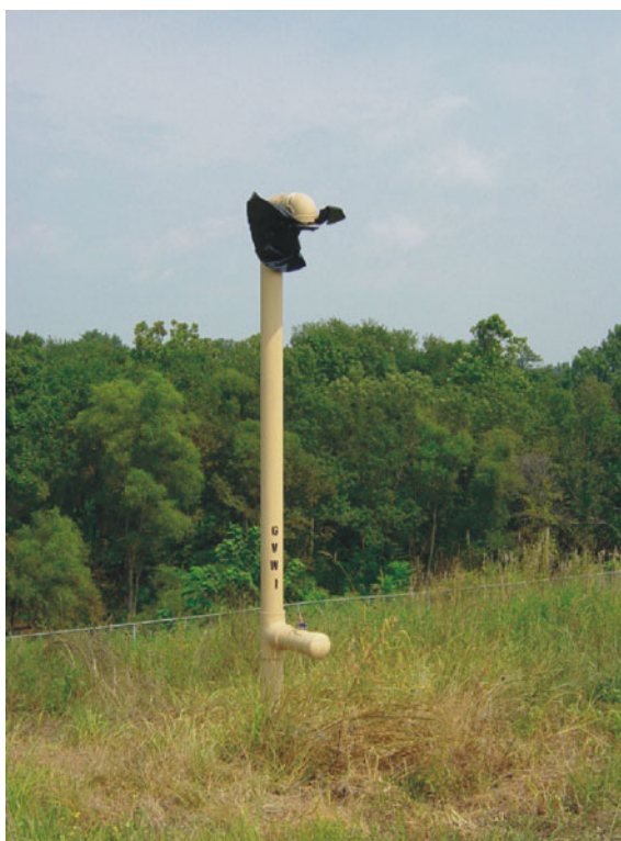
Passive Vent on the Top of the Bush Valley Landfill
