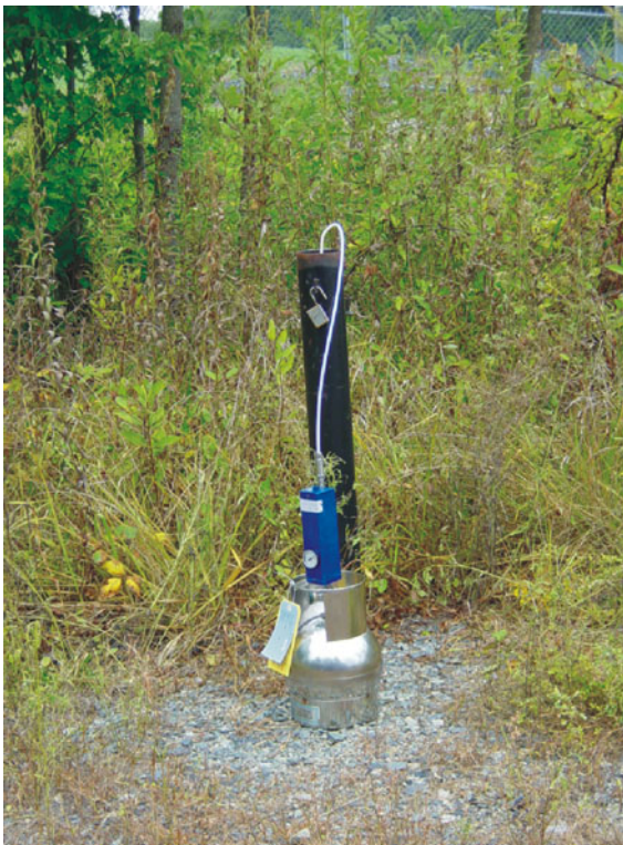
Landfill Gas Sampling at a Perimeter Gas Monitoring Probe
