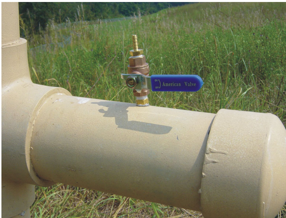
Sampling Valve Installed on a Passive Vent
